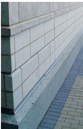
Masonry raised above grade
