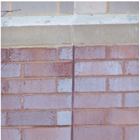
Figure 7: Change sealant color within the vertical joint to match changing unit colors up the height of the wall.
