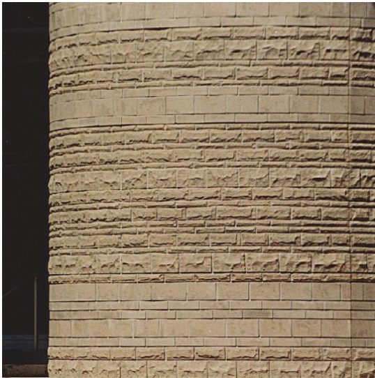
Figure 6: Sealant colored to match color of adjacent veneer units.
